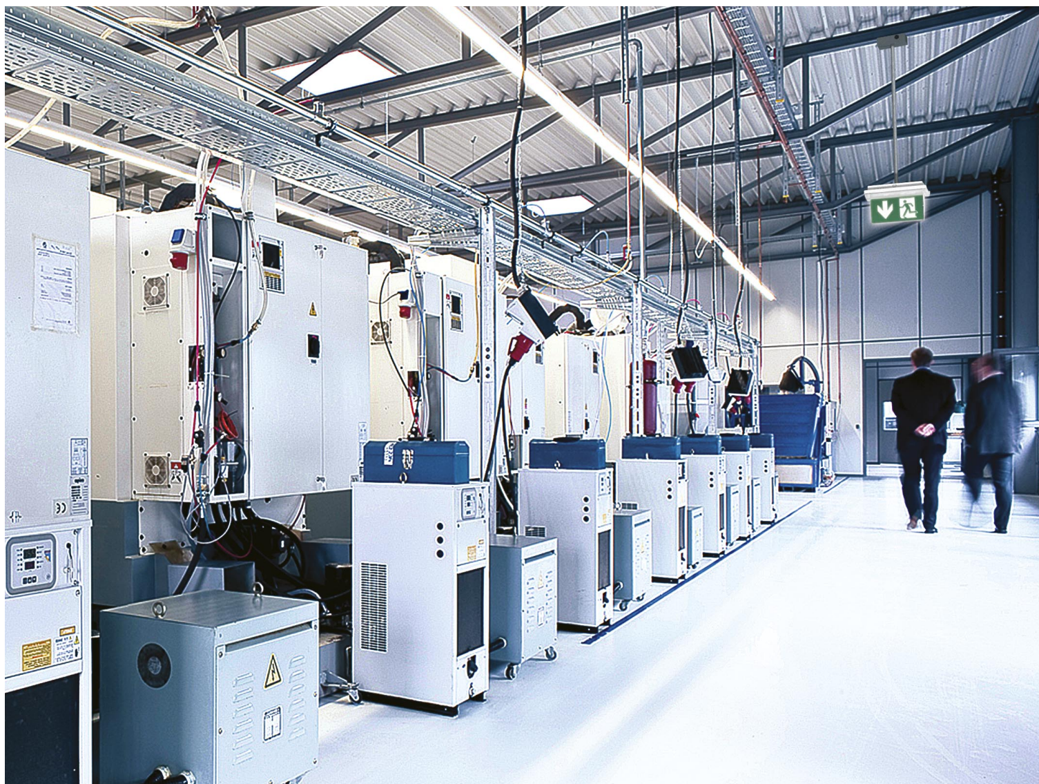
Industrial Area Emergency Lighting Application
